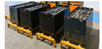
~1500 V energy storage
